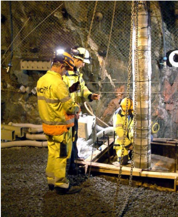
Installation of one of the three parcels illustrating the mixing of the different compacted buffer discs.
